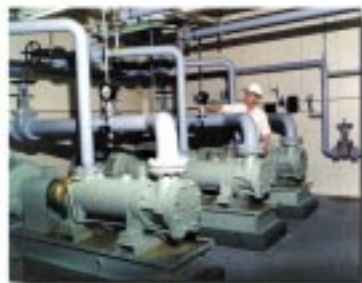
Three 1/2 capacity 8L-400 pumps delivering fuel oil to power plant boilers
