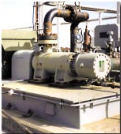
8L-630M crude oil pipeline pump in Western Canada delivers 900 GPM at 1440 PSIG, 1200 RPM, 1000 HP
